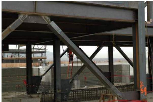
Fig. 13. Star Seismic WildCat braces used in inverse V (foreground)
