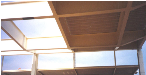
Fig. 1. Construction of I beams gird of h=2000 mm having bolts butt connections subjected to experimental investigations
